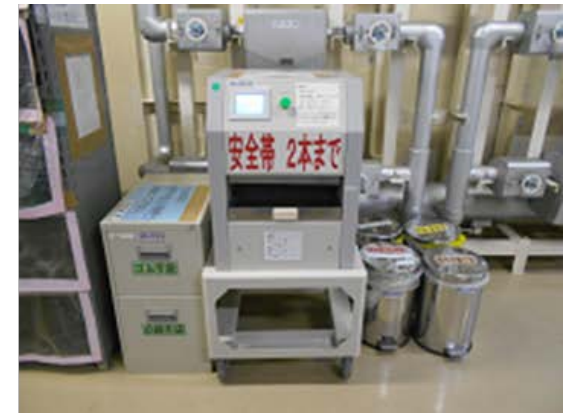
7 PPE monitors in unit-3 RCA
